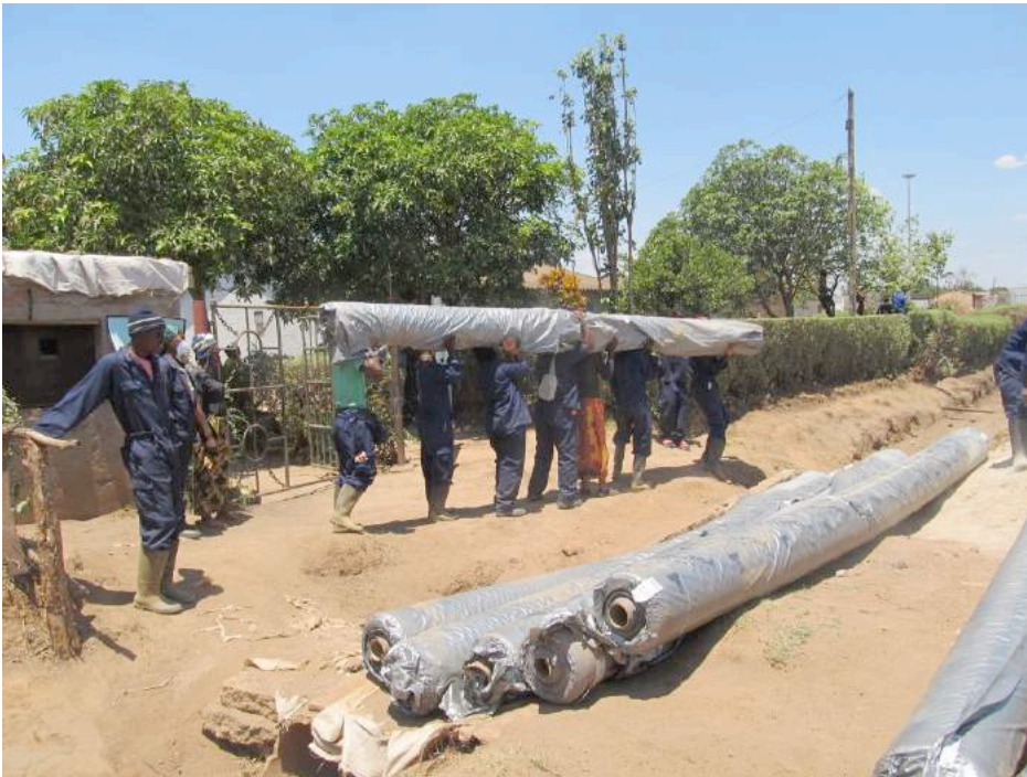
Above: A remediation team carries a rolled up barrier cloth, also called a geotextile layer, into the yard of a home to prepare it for encapsulation
