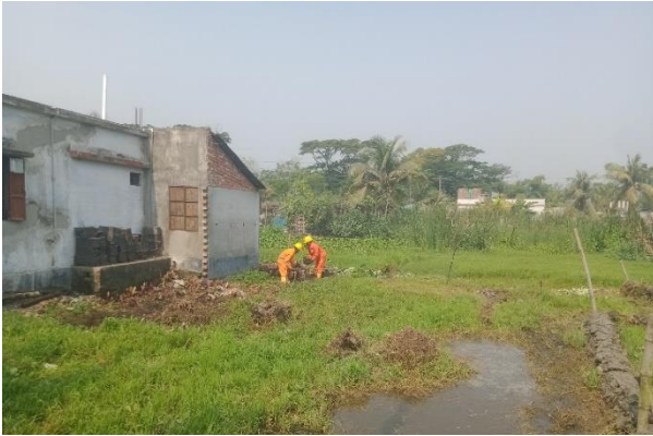
North dumping site before remediation work
