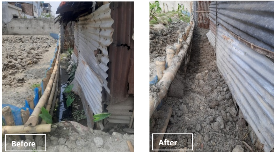
Figure 53: Waterlogging issue due to the capping work in the South site of the West dumping site.
