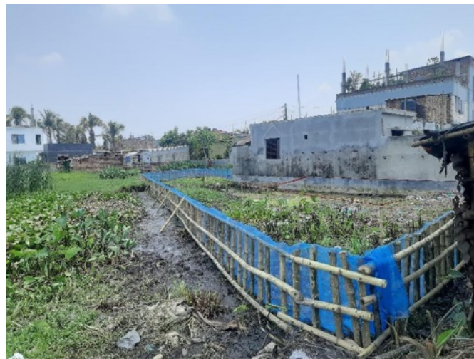
Figure 21: Bamboo piling work in the North and West side of Mr. Badi's house.
