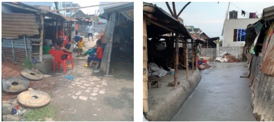
Figure 33: Road and house yard brick soling area before (left) and after (right) concrete work.
