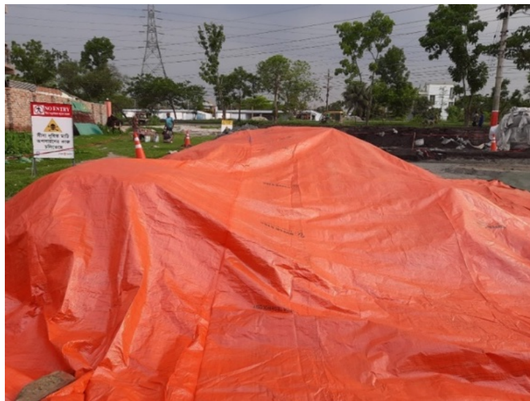
Figure 40: Tarpaulin was used for covering the excavated clean sand stockpile of the south dumping site.
