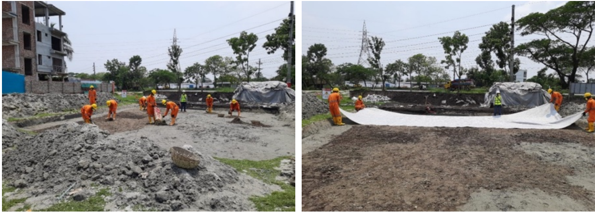
Figure 41: Placing scrapped contaminated soil and geotextile marker layer in the South dumping site.
